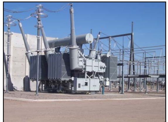
Large power transformers with extra-high voltage ratings will be the first products manufactured at Mitsubishi Electric Power Products' new Memphis factory.
